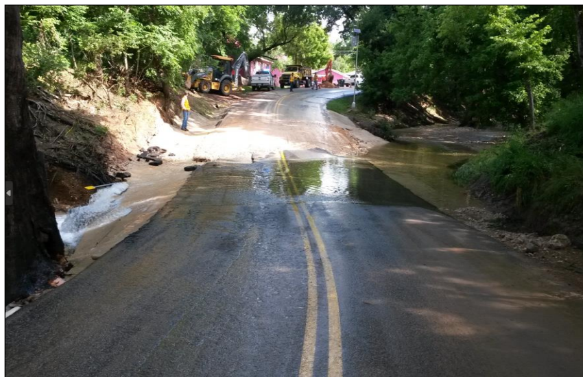
Figure 3: June 2016 Post-flood Photo of River Road crossing
